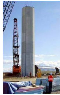
A silo liner being lifted into place for installation into a missile silo at a launch complex under
