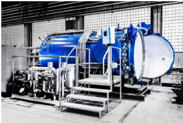
Autoclave system for UF 6 feeding
